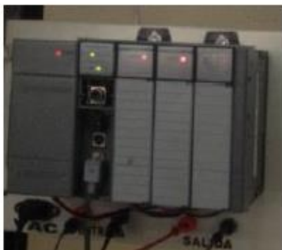
Figura 5. PLC Allen Bradley SLC500
